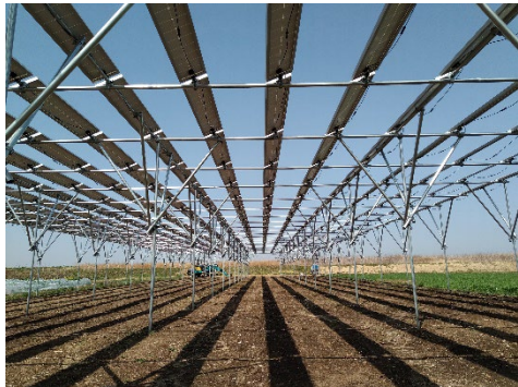
DC 65 kW (low voltage) APV
