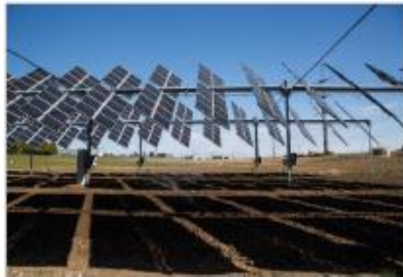
Figure 8: Agrolvoltaico® plant in France (2019)
